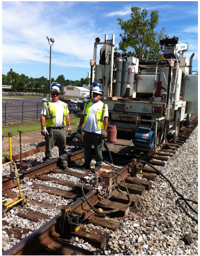
Right: A crew of two weld a joint on the NEW heavier rail recently installed through downtown Madisonville at the Center Street crossing. 7/8/14 -Bill Corum
